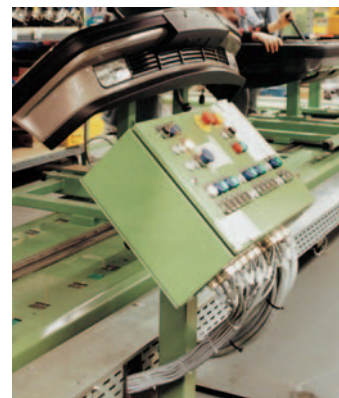
Measuring and control cables in automobile factory.
